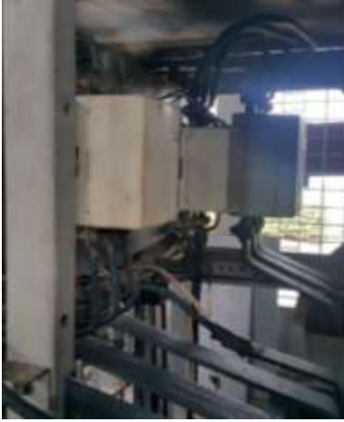
Fig.15.Magnetic contactors and Busbar
